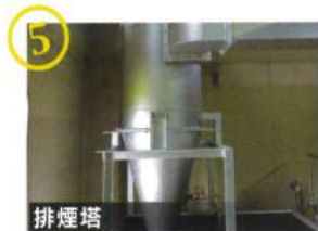
Exhaust Gas Collection by Water Scraper
